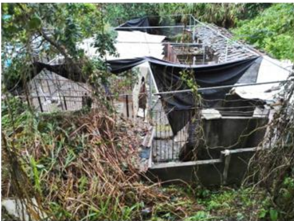
The top of the shelter was seriously destroyed
